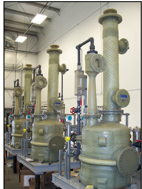
Client: AREVA NP Lynchburg, Virginia
